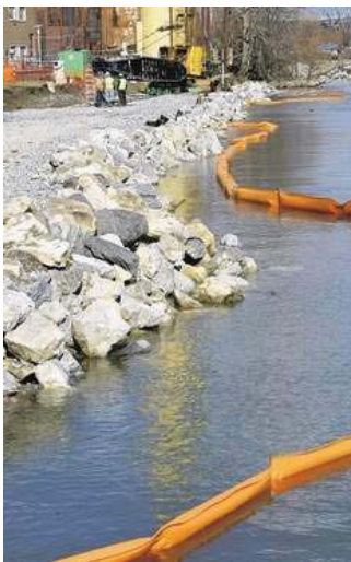
A floating coal-tar containment barrier off the Hudson shoreline near the Newburgh water treatment plant will be replaced by a permanent containment wall. Times Herald-Record/JEFF GOULDING
