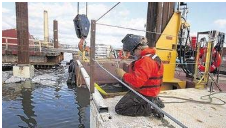
Welder Steve "Shorty" Haviland of Cambridge works on a barge in late January as part of the Hudson River coal-tar cleanup. Times Herald-Record/JEFF GOULDING
