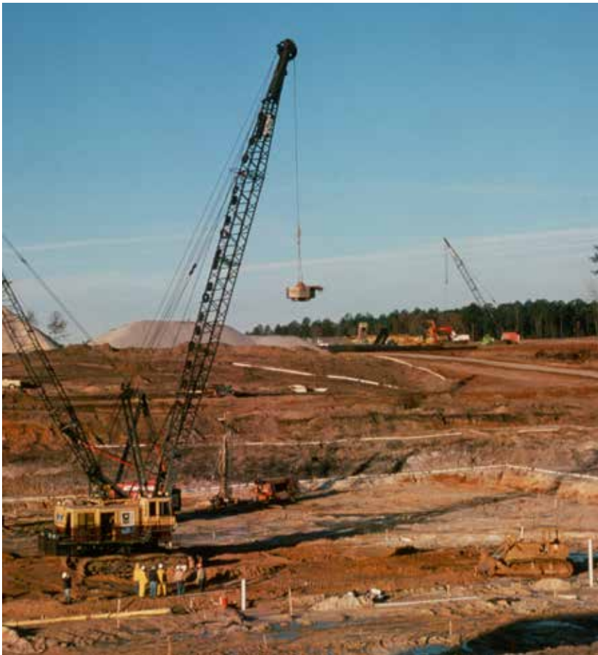
Dynamic compaction of foundation soils for Steel Creek Dam at the Savannah River Plant, SC.
