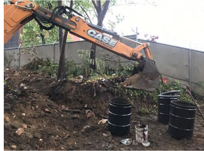
Photograph 10: Released black viscous oil and impacted soil was excavated and placed into 55-gallon drums for off-site disposal. Date: August 7, 2017.
