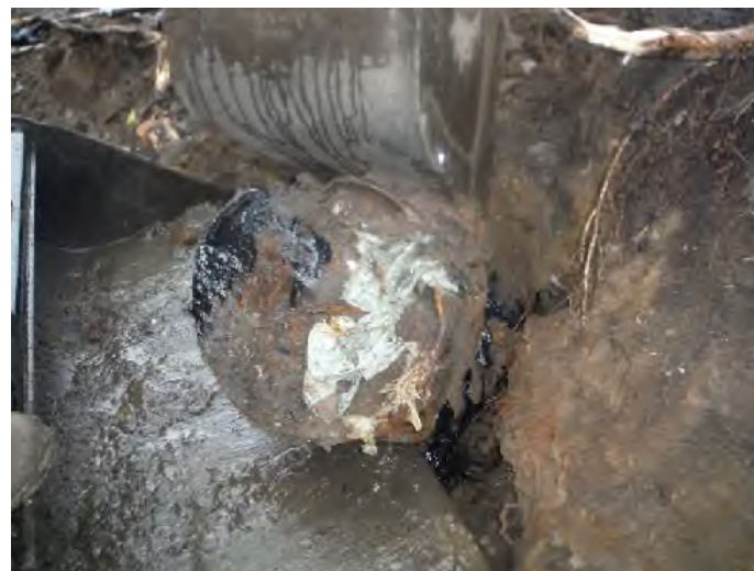
Photograph 8: During re-grading activities, a buried 55-gallon drum encountered and punctured . Contained a black viscous oil. Date: August 7, 2017.
