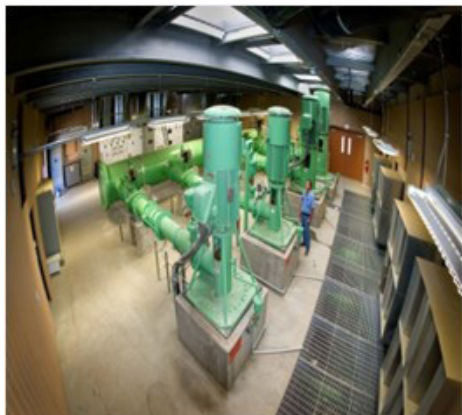
4. Thomas E. Levy Groundwater Replenishment Facility, Coachella Valley Water District .
